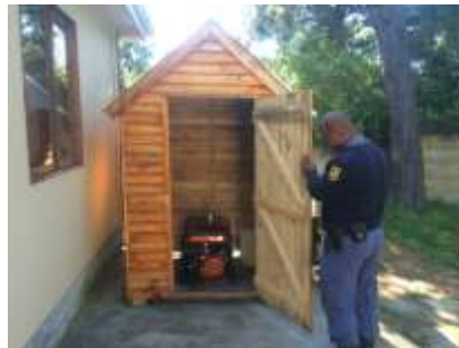
Eishkom backup generator shed
